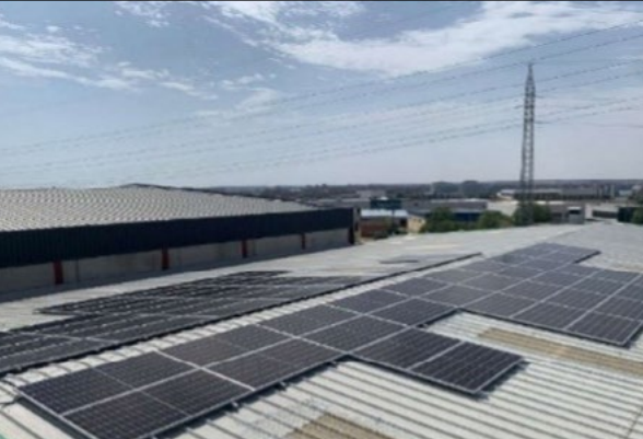
Solar panels at Intersurgical Spain
